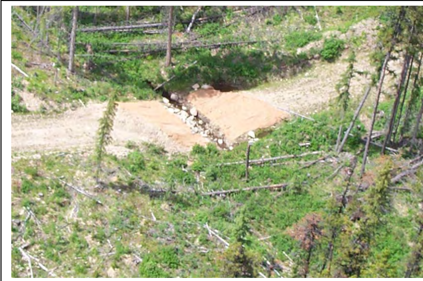
Photograph # 1143: De-activated crossing W08
