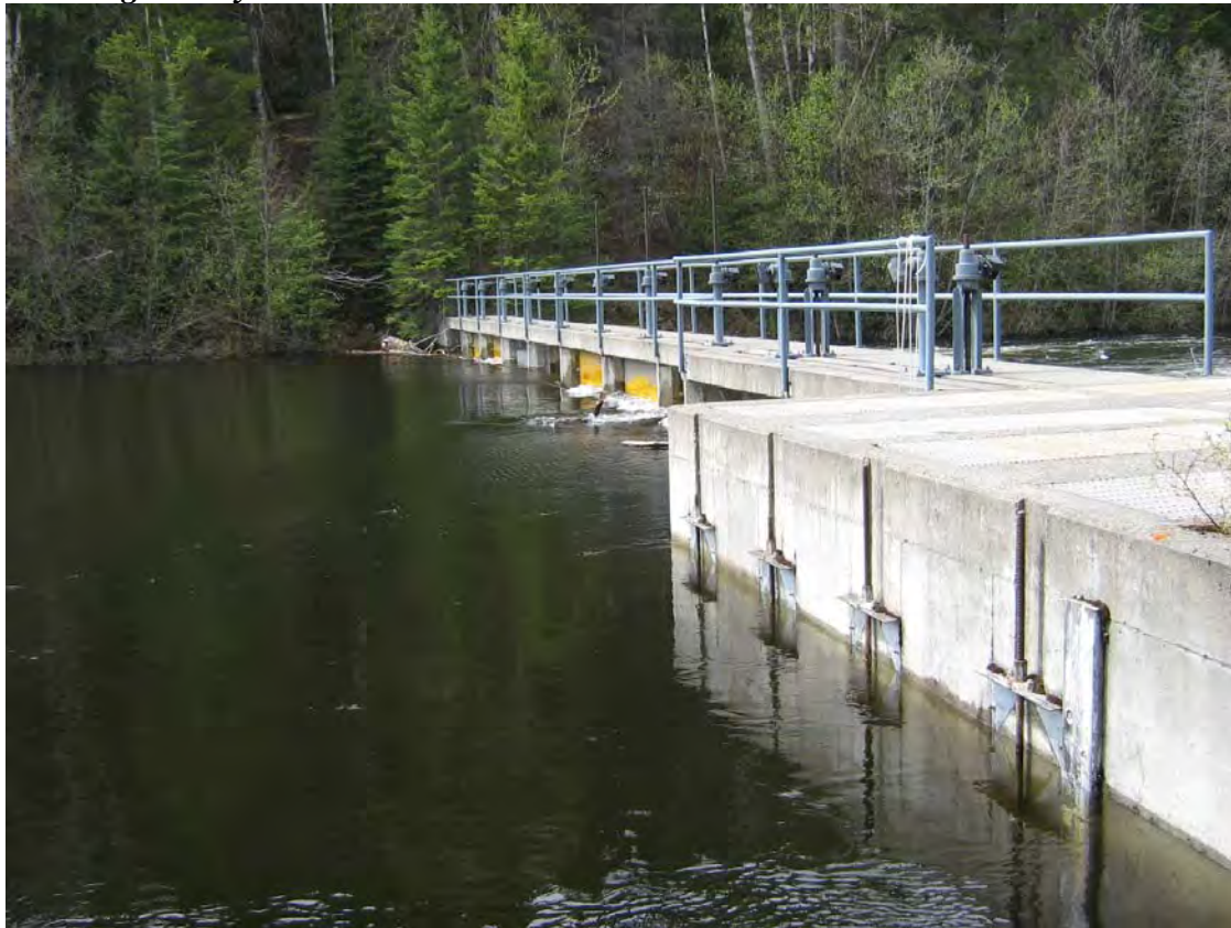
Figure 9: Upstream view of McKinley Dam with fishway on the right. Water storage occurring in May 2008.
